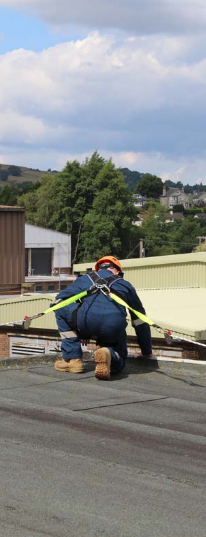
MATS Rooftop Worker - Safety Access
